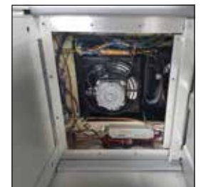
A5. Condenser compartment
