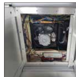
A5. Condenser compartment
